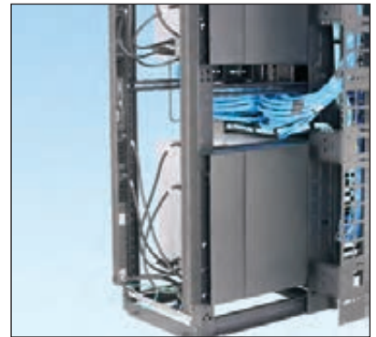
Panduit 4 post rack thermal ducts shown in a dual Nexus 7009 switch deployment.
